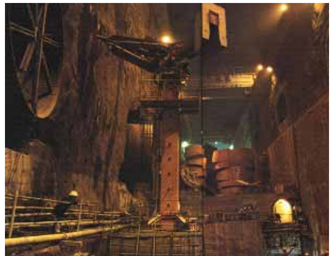
Turbine / Generator Hall excavation (cavern: 252m long, 26m wide and 61m high)
