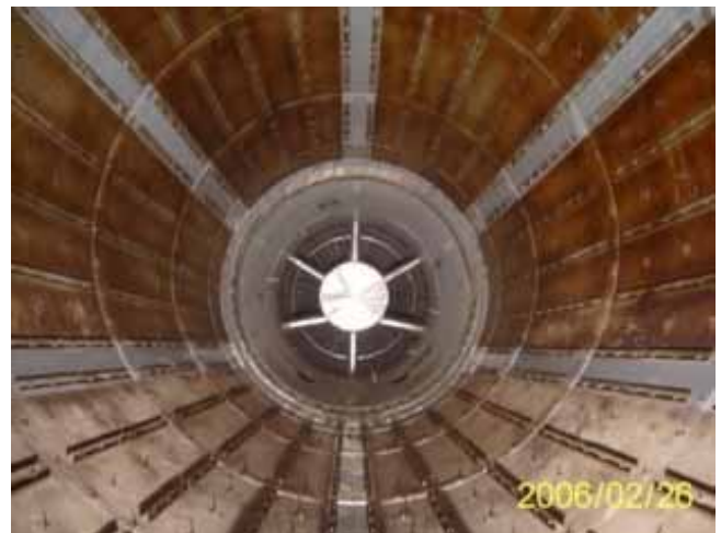
Internal View of Unit 3 Bypass Stack
