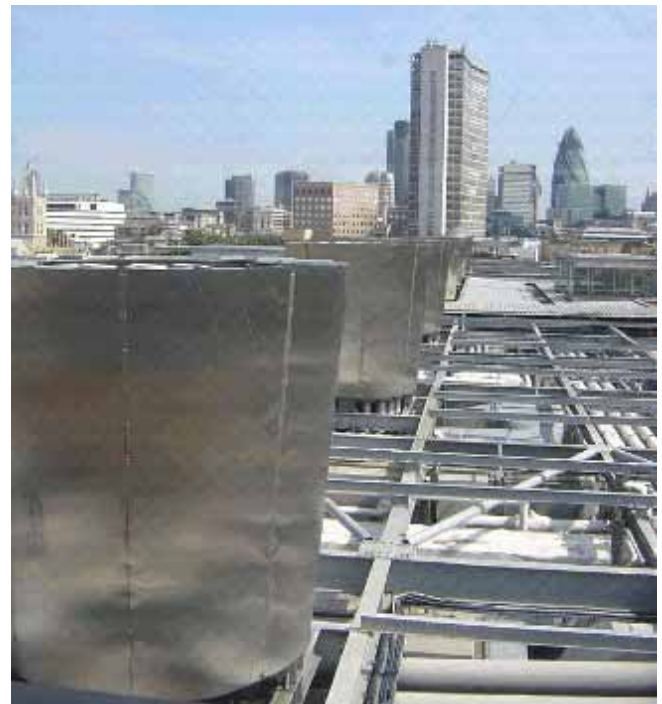
HVAC equipment on roof of New Hunt's House
