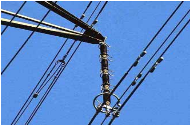
High Voltage Electricity Transmission Pylon
