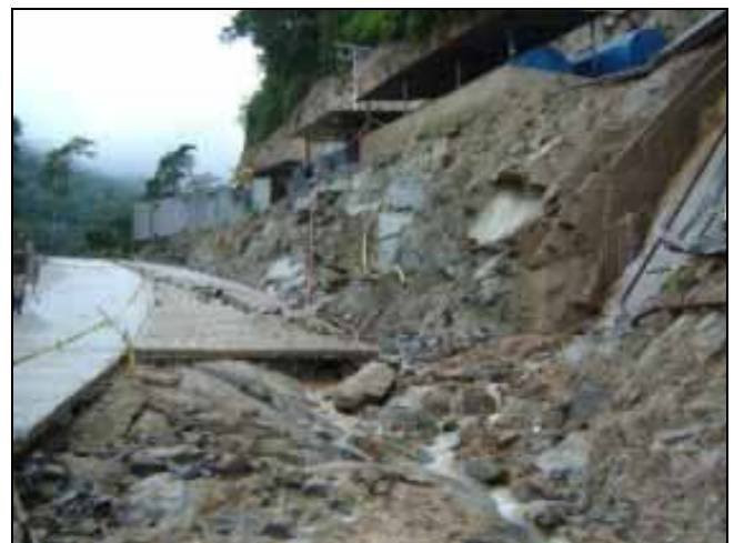
Damage to Access Road as a result of the storm
